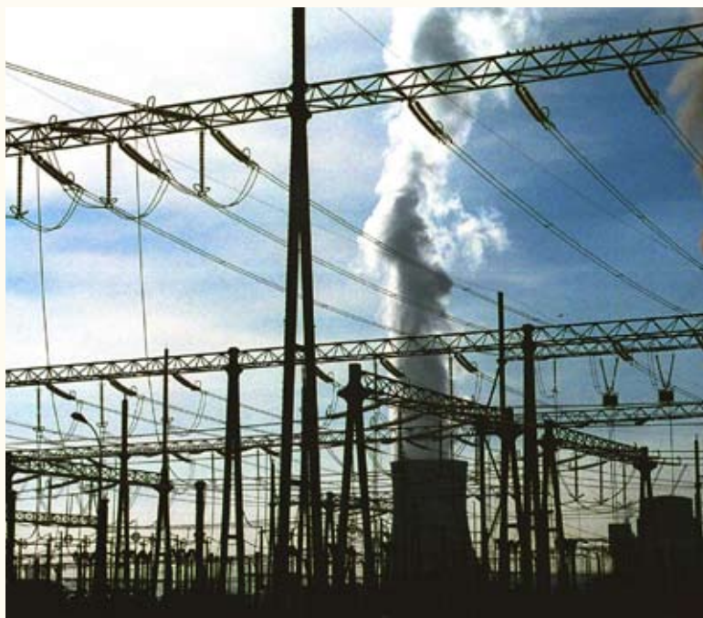
Hot wires – Transformer station and cooling tower of KEK power plant “Kosovo B”
